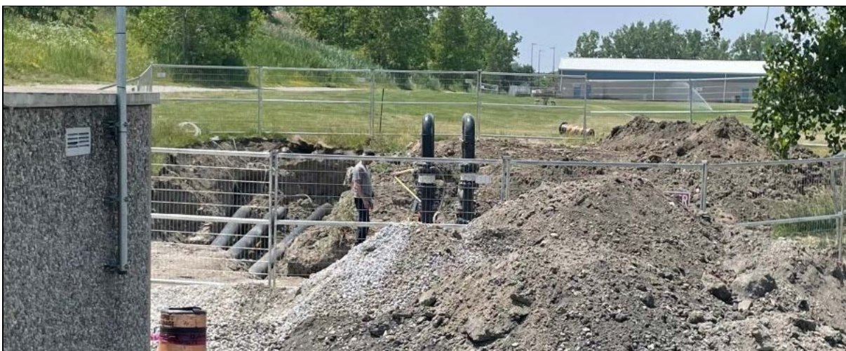
Construction in Malden Park, Windsor, Ontario to expand pipeline network and brine wells for extracting and transporting salt brine to Windsor Salt's evaporation plant
