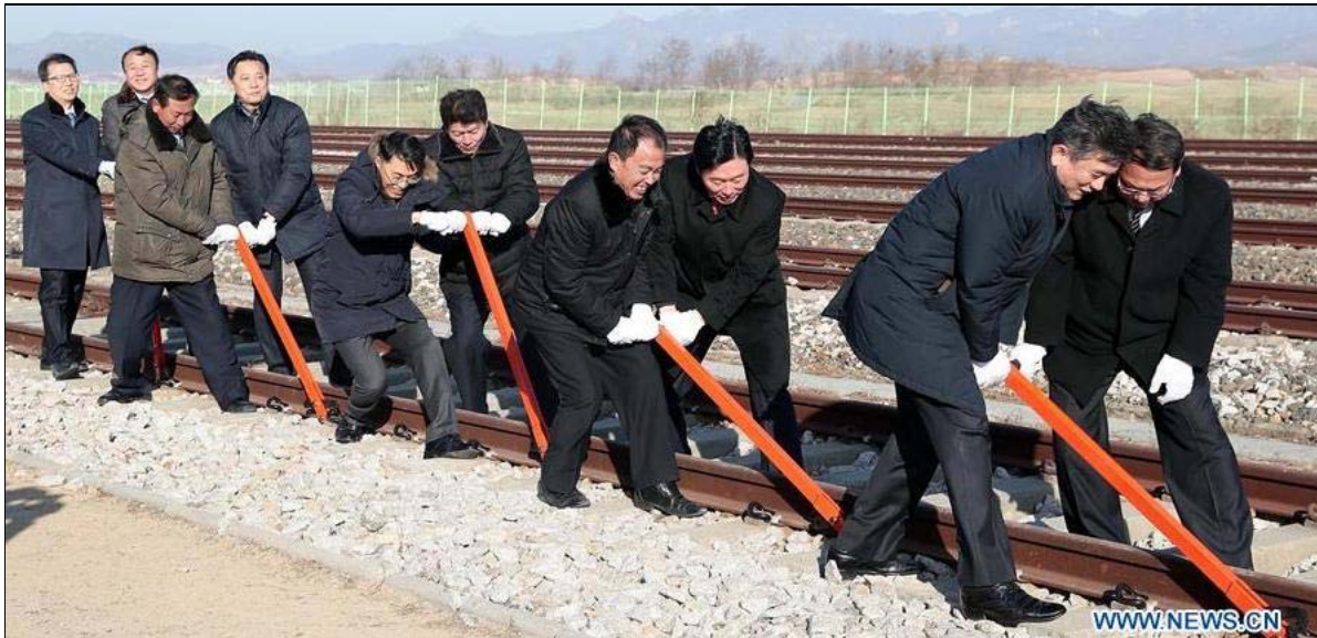
Officials from the ROK and DPRK connect the rails from north and south.
